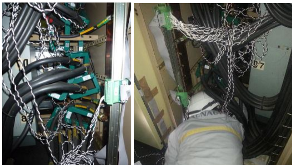
Figure 2. Internal sight of an electrical cabinet with sensors of current
